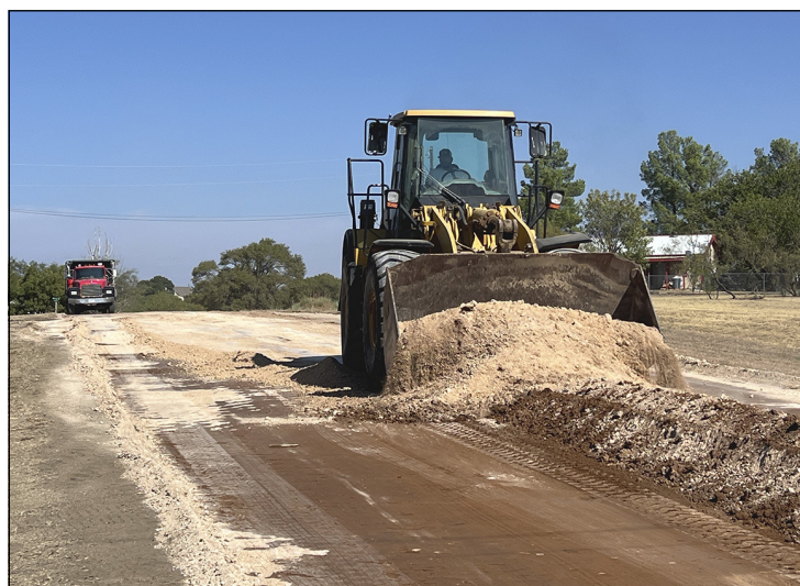
Road Work Ahead G&G Operators have been working hard on the rehabilitation of a section of Rick Husband Boulevard in Howardwick. Work began on the project last Thursday, and officials say they hope to have the road finished by the end of next week. Traffic is being diverted to other routes in the city while construction is underway. ENTERPRISE PHOTO
